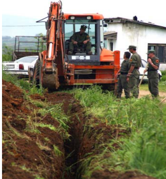
Construction of community water supply network for 7 ethnically mixed villages in Prizren Municipality
